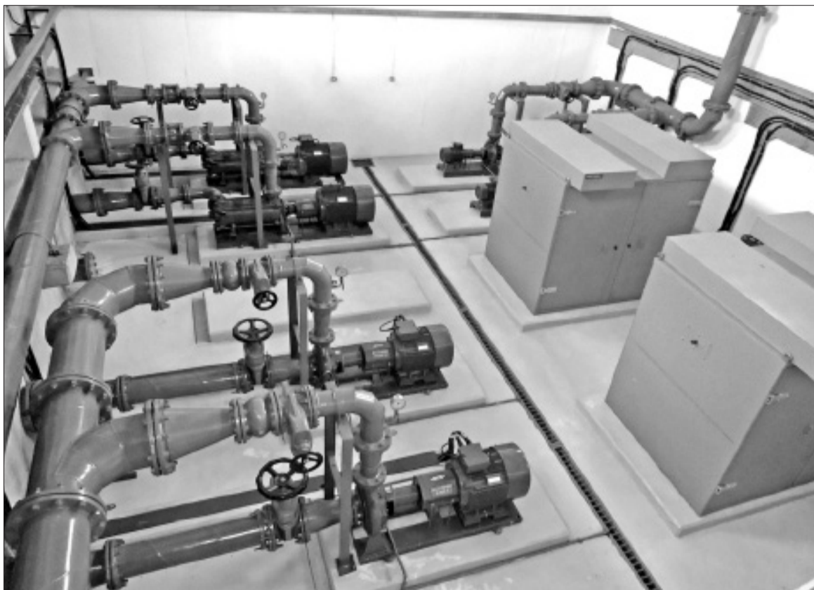
Horse pipework at Nyewasco water treatment plant at Kamakwa at the outskirts of Nyeri town. Photo/Joseph Mukubwa
