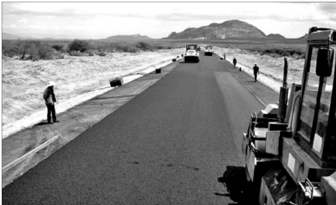
Workers of China Wu Yi construction company tarmacking the 136 kilometer stretch of the Isiolo-Moyale road, which is projected to be complete in September three months before deadline in December 2010. Photo/Hussein Saleasa
