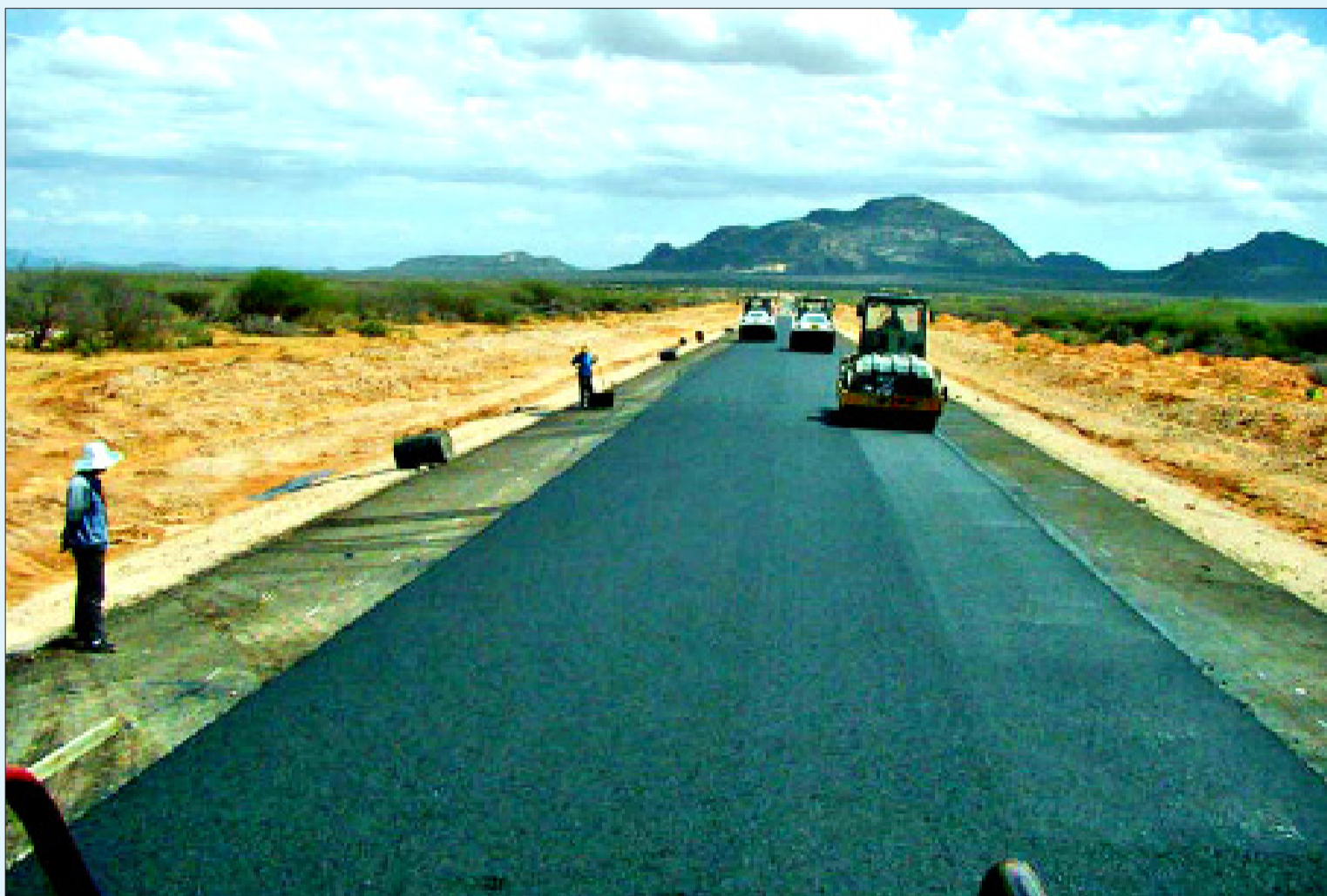
A section of the 136Km stretch of Isiolo Moyale road which is under construction. The road is expected to be completed by September this year. Photo/Hussein Salea
