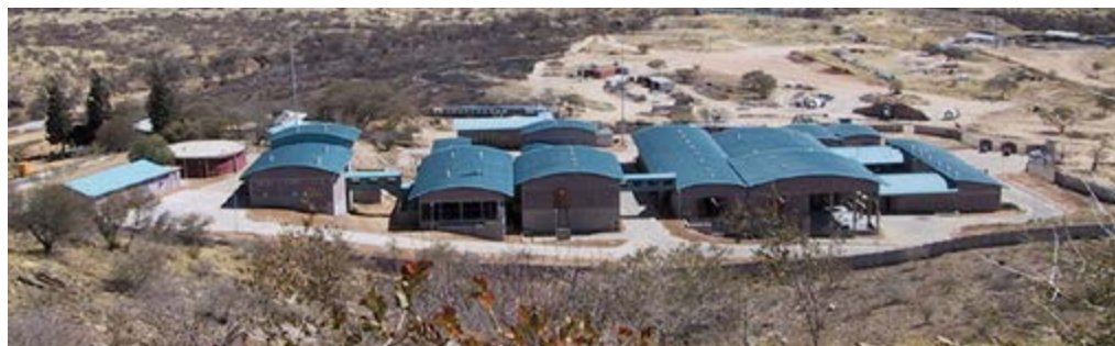
Figure 11: Windhoek's water reclamation plant [Source: P Heyns]
