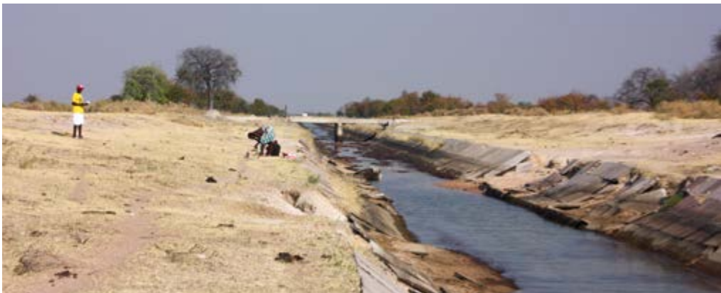
Figure 44: Dilapidated water infrastructure in north-central Namibia [Source: G Schneider]
