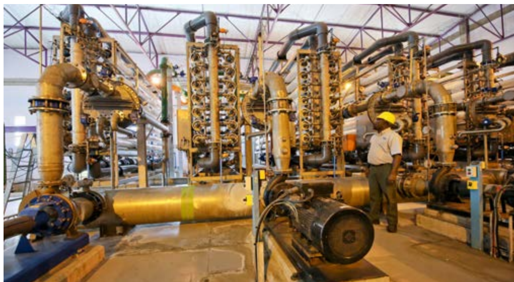
Figure 19: Ultra-filtration at Windhoek's water reclamation plant [Source: G Schneider]
