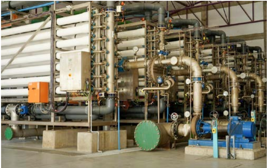
Figure 137: Carbon filtration at Windhoek's reclamation plant [Source: Veolia]
