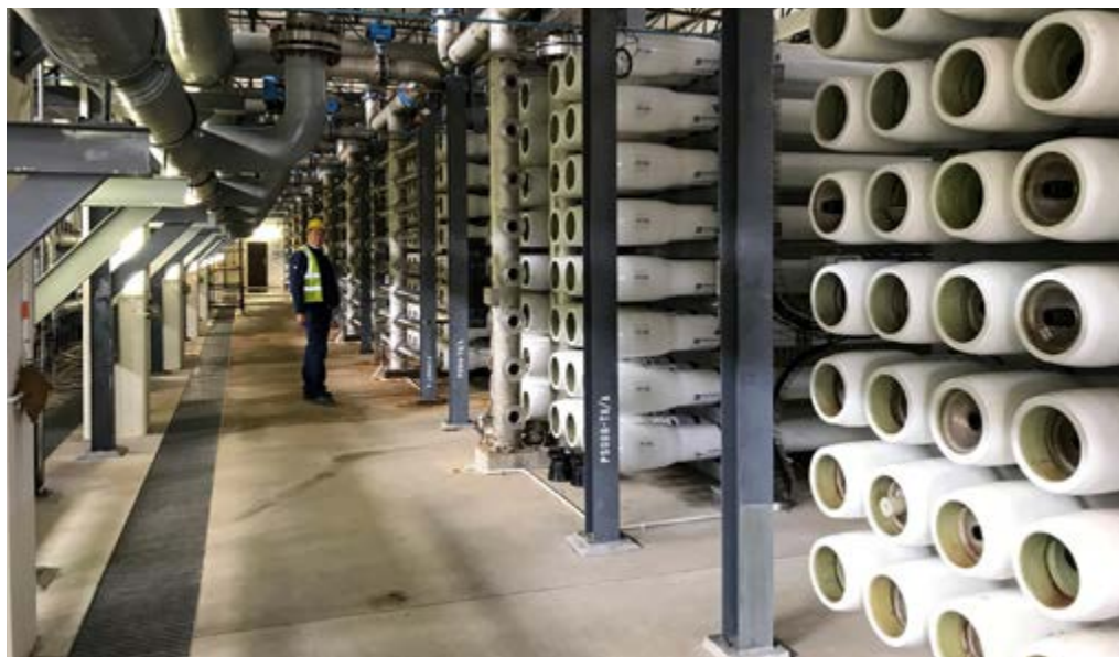
Figure 13: The Erongo Desalination Plant's reverse osmosis assemblies [Source: G von Oertzen]
